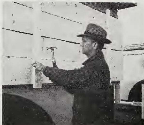
The boarding up of box offices, concession buildings, etc., will keep these areas safe from the weather, and help discourage breakage and theft.
